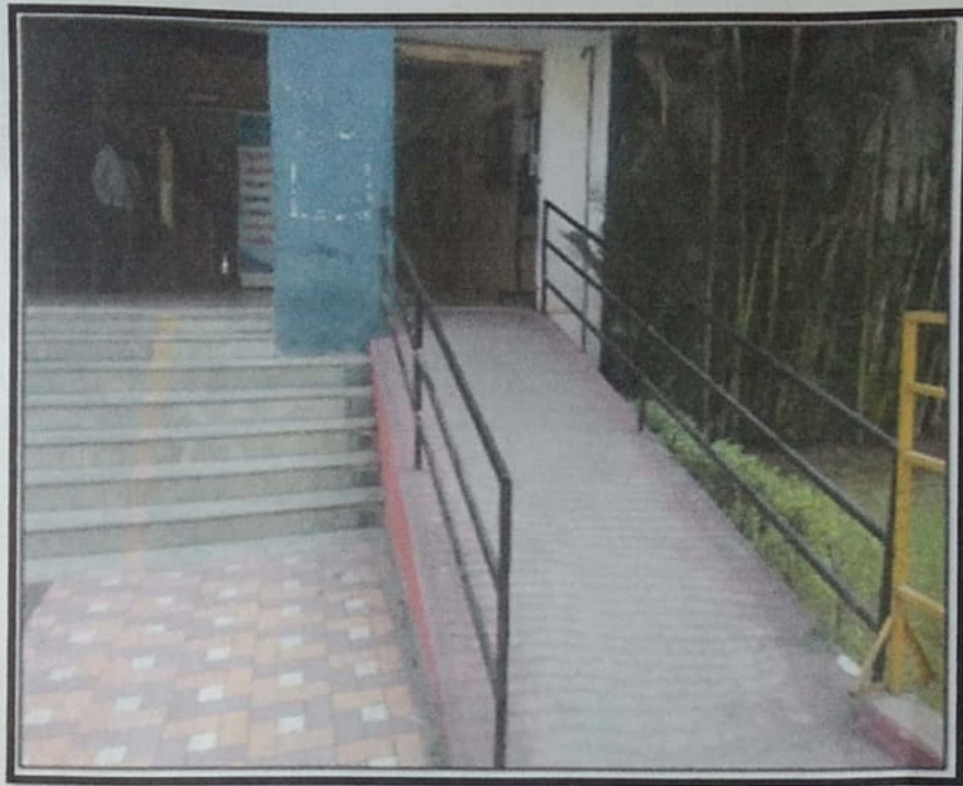
Ramp for Physically disabled
