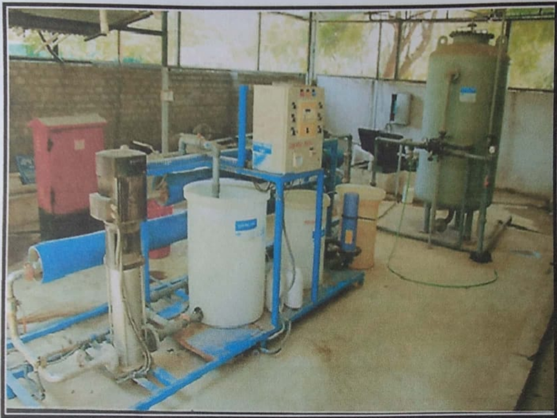
Water Purification Plant
